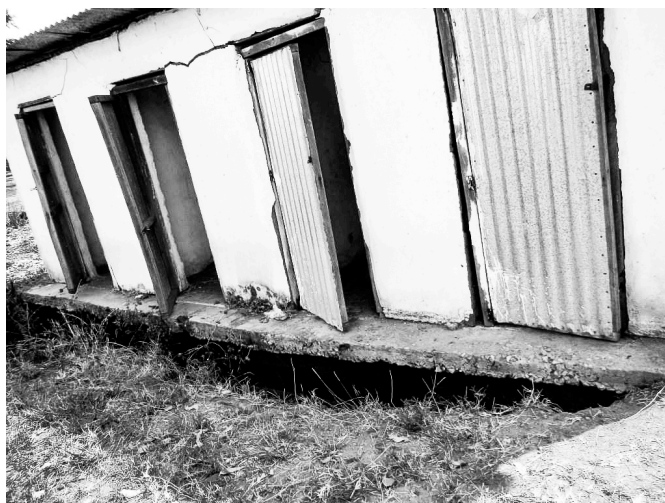
Above: Restroom outside of a school in the capital city of Juba. Growing sink hole results from a lack in maintenance.
