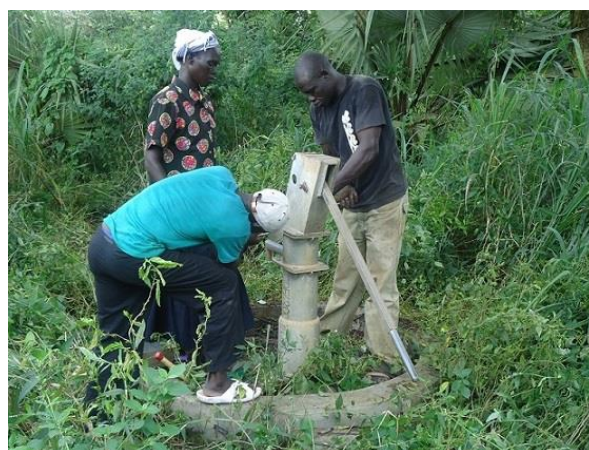
Above: A broken borehole
