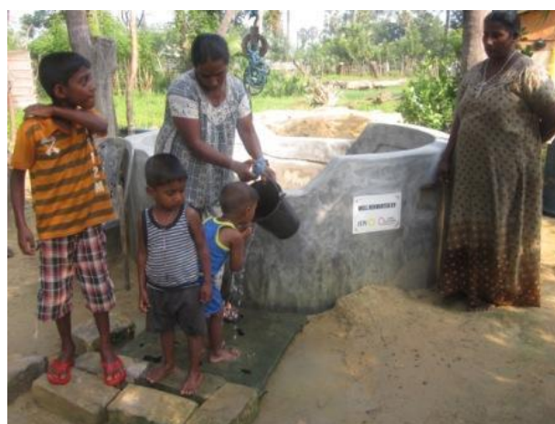
Above: Renovated well at Ms. Toffek's household being used to provide drinking water
