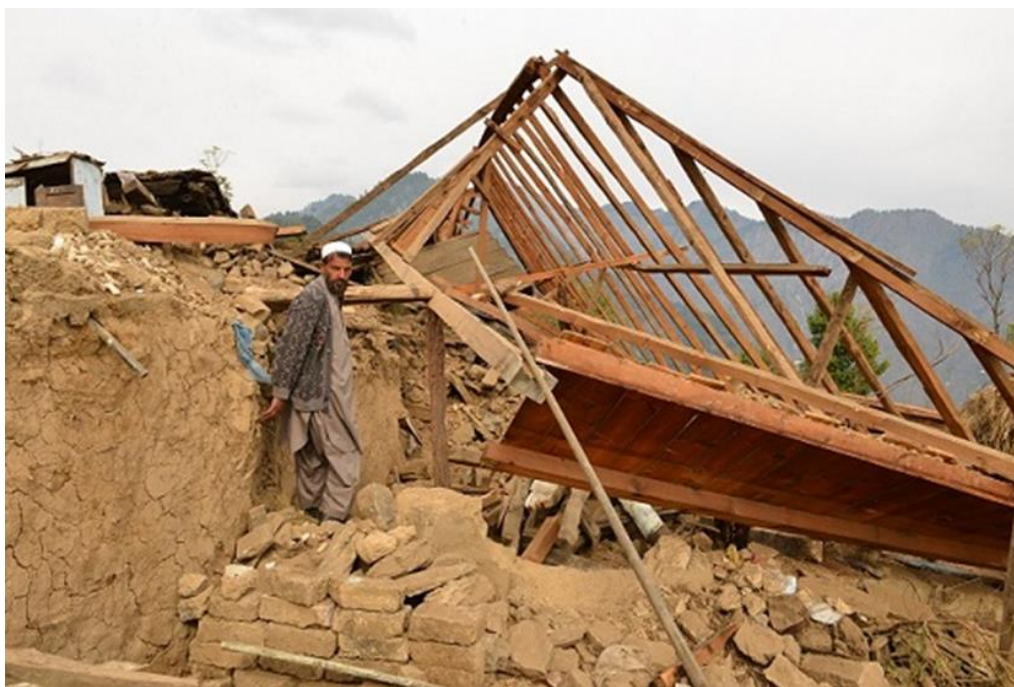
The aftermath of the earthquake in Shangla district in Pakistan
